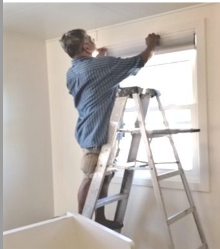
← Adrian Daligcon installing window shades in the Pastoral Center; assisted by Roger Isidro .
