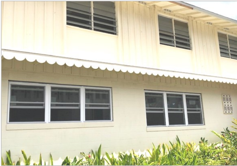
Photo 2: The difference between the old jalousie windows in the second level and the new up-down slide glass panes in the ground level during installation.
