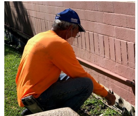
Rudy Fiesta sealing the leaks for rainwater on the concrete wall of the church. Together with Roger Isidro they worked on the interior and exterior walls of the sanctuary and afterwards fixed the bells on the belfry.
