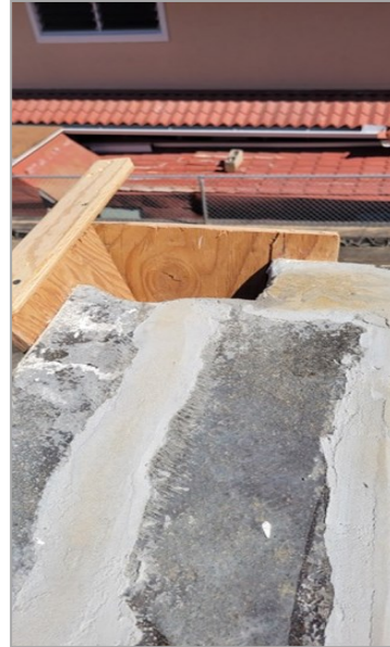
(Photo at left); The cracks on the concrete roof of the hall kitchen being repaired by Rudy Fiesta , Carlito Centino and supervised by Roger Isidro .
