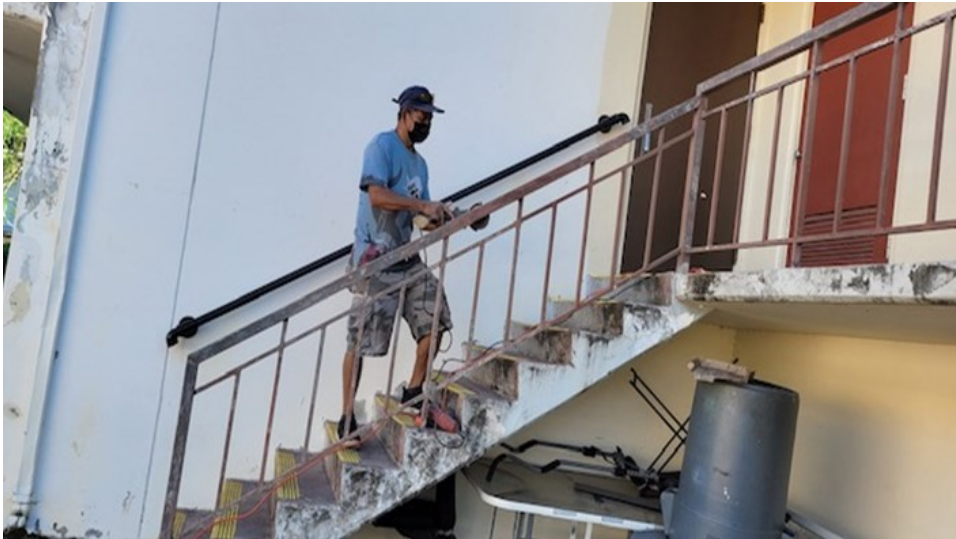
<Carlito Centino repainted the guardrails of the staircase to the hall kitchen
